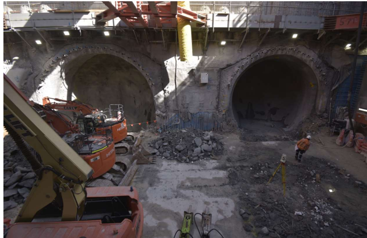
The two stub tunnels at the Eastern Portal retrieval shaft, South Yarra
