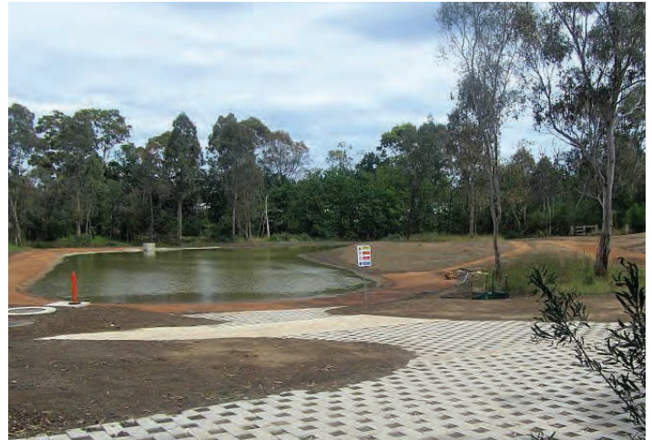
Figure B4.3 Bolin Bolin integrated water harvesting wetland post-construction in 2018
