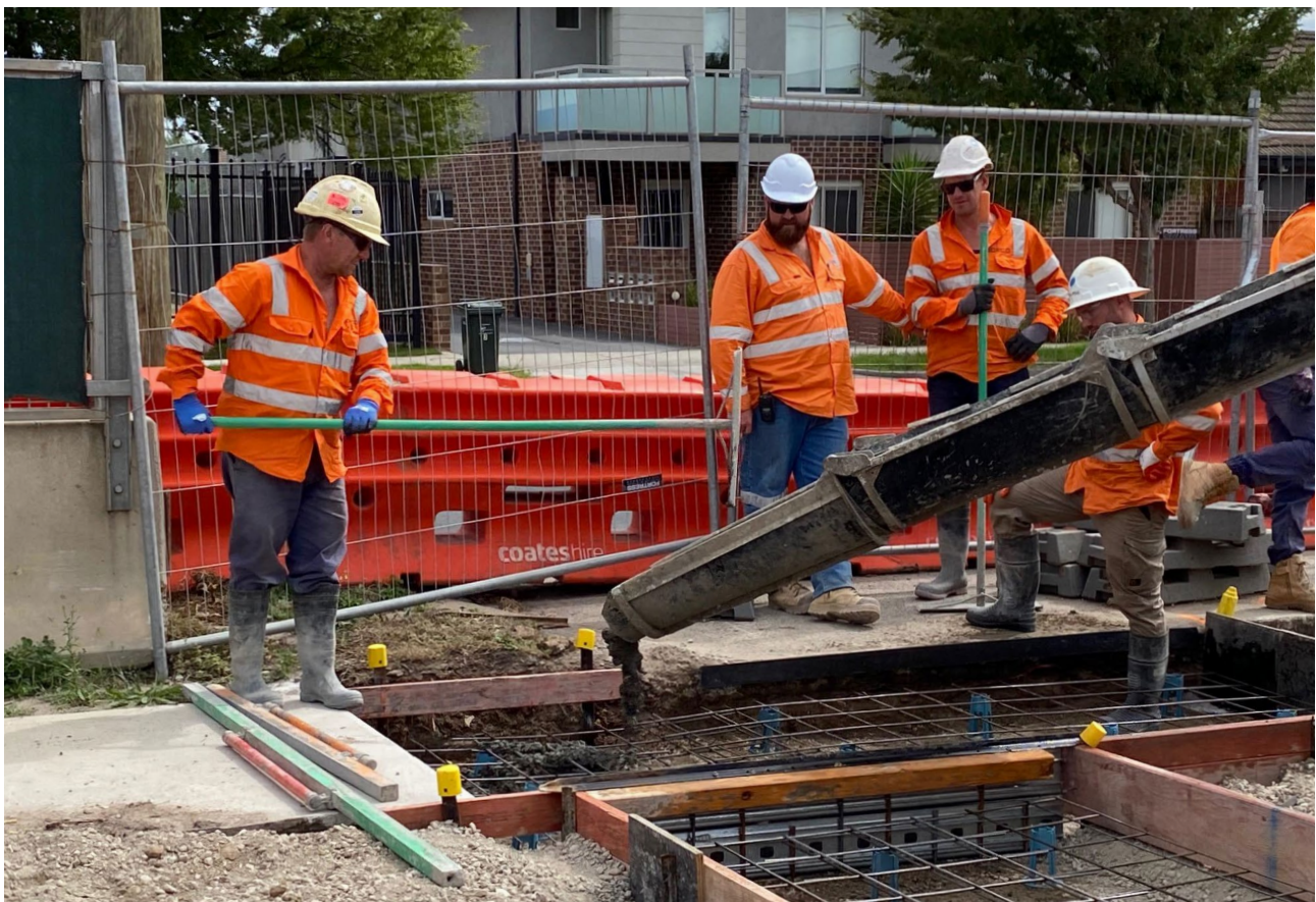
Figure 60. Unwashed recycled glass fines concrete pour at Reservoir station Shared User Path (SUP)
