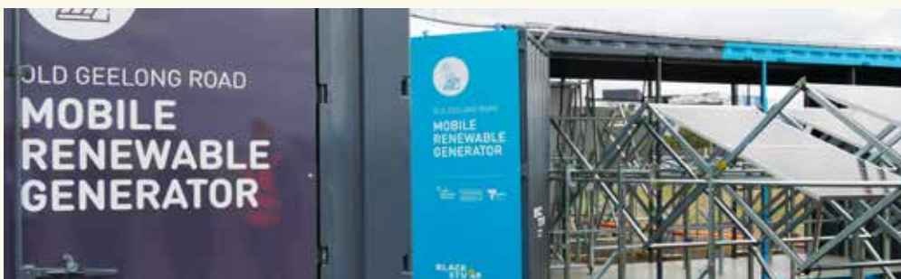
Mobile solar unit at Old Geelong Road
