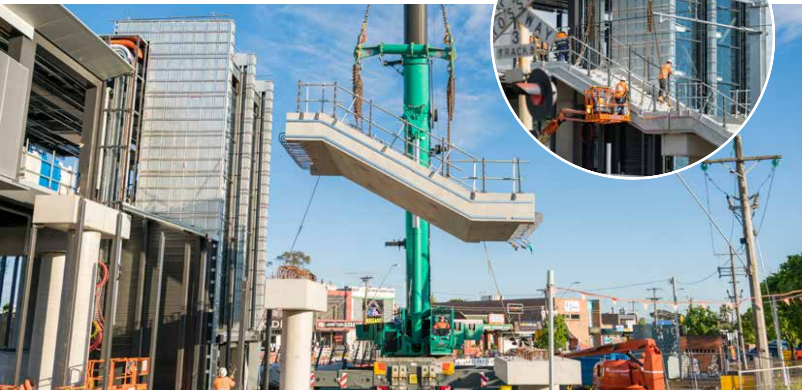
Below and right: Installing the northern stairs for the new pedestrian and cyclist overpass
