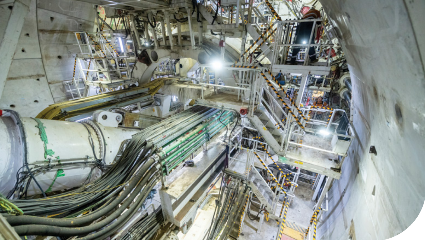
TBM Vida pushing the cutting head forward and laying concrete rings behind
