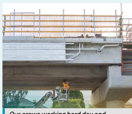
Our crews working hard day and night to complete the rail bridge by early August.
