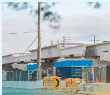
Concrete u-troughs installed on top of piers for the rail bridge structure.
