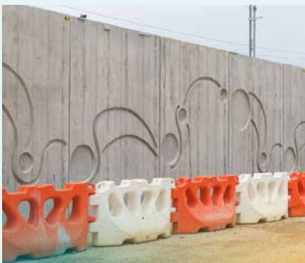
Progress on the retaining walls on the southern side of the rail bridge.
