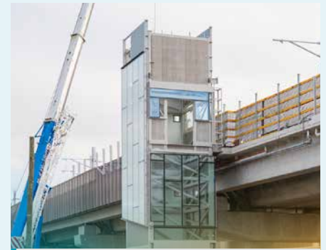
The first lift shaft, out of a total of four, being installed for passengers to access the elevated platforms.
