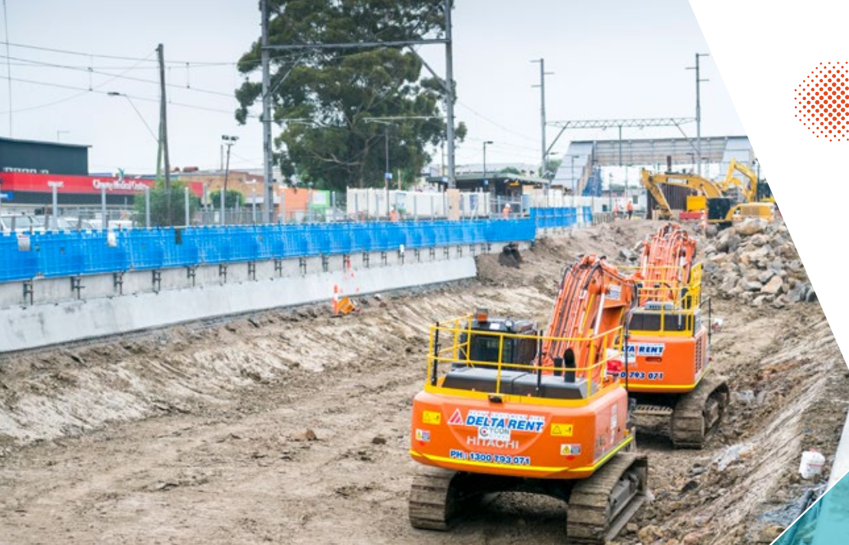
Excavation the rail trench on the Glenroy Road Level Crossing Removal Project.
