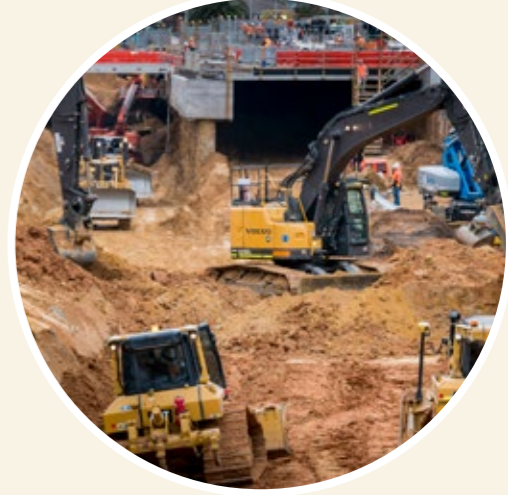
Top circle: Mont Albert Road level crossing. Bottom circle: This excavation in Cheltenham is similar to what's required at Surrey Hills and Mont Albert.
