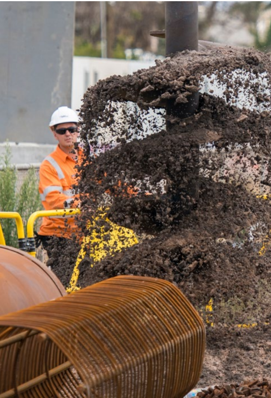
A combination of sheet piles and continuous flight auger piles (pictured) are being installed across Edithvale, Chelsea and Bonbeach
