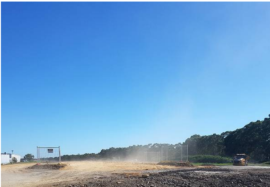
Left: Wind blown dust after a truck had passed – north of Park Way entrance. It was noted that the section of the access road south of the Park Way entrance appeared damp, while the Park Way entrance and the section north of the entrance appeared dry and truck movements generated significant dust.
