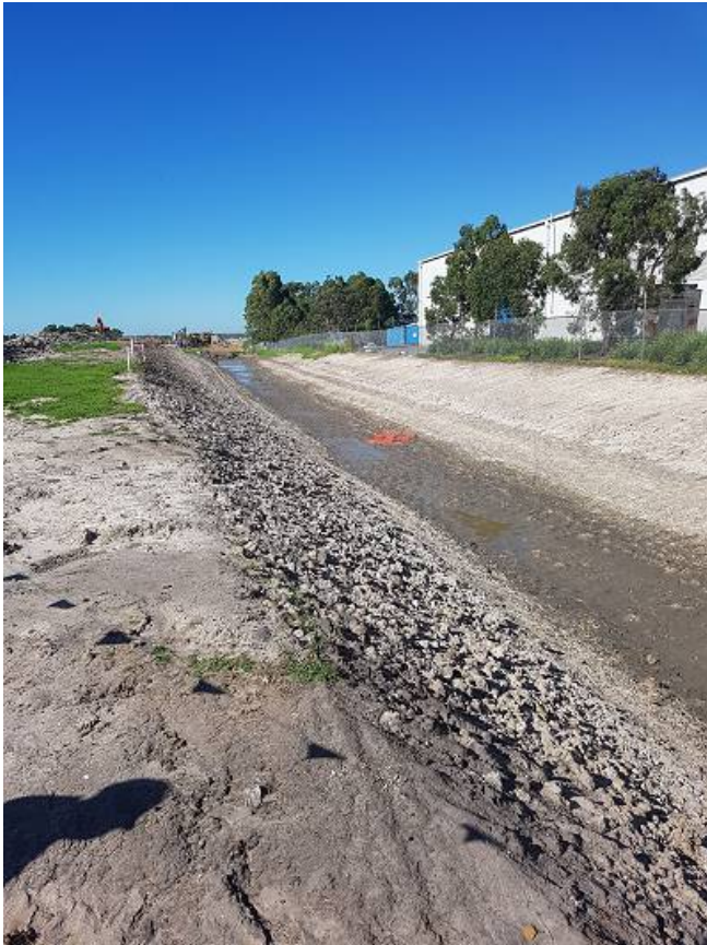
Left: An example of one of the large swales used to successfully contain storm water run-off during normal rain events over the summer period.
