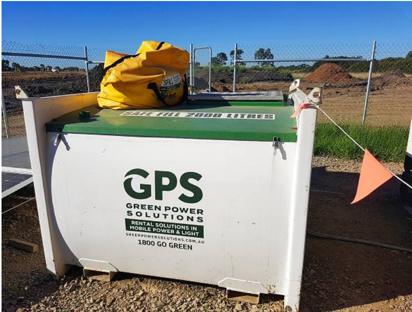
Left: Spill kit on the Governor Road generator fuel tank, ready for use in case of a spill during refueling.
