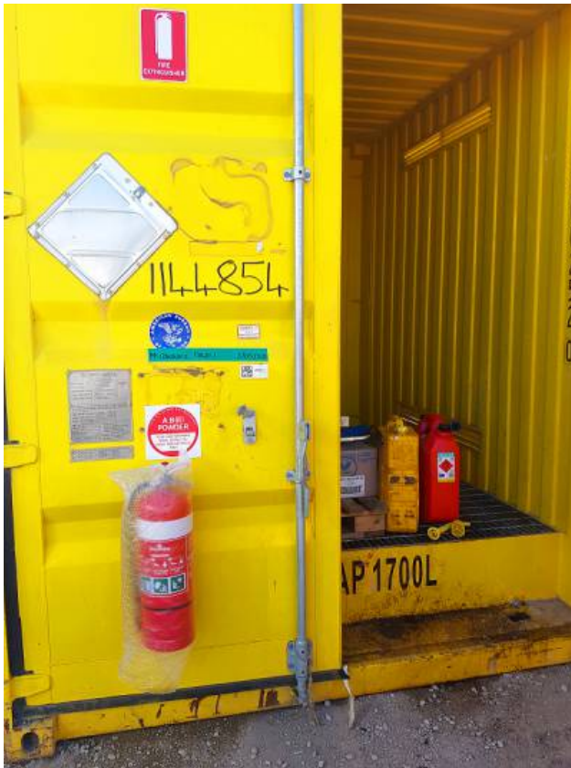
Left: The flammable goods container at the Governor Rd Compound. Note the missing DG diamond. Also note the close proximity of the fire extinguisher to the flammable materials. This would make it difficult to access the fire extinguisher in case of a fire.
