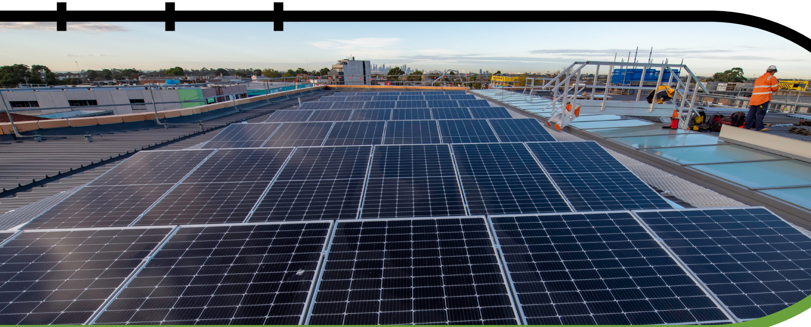
Solar panel system. Subject to change.
