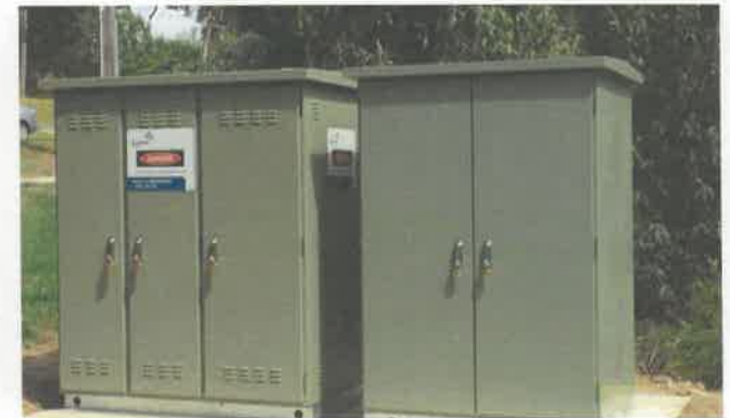
Figure 35. Typical steel cabinet HV kiosk
