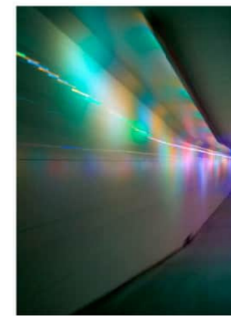
DEMONSTRATES LIGHTING THE VERTICAL ELEMENTS OF THE UNDERPASS TO IMPROVE VISUAL COMFORT, WHILST MAINTAINING COMPLIANT AND LIGHTING LEVELS.
