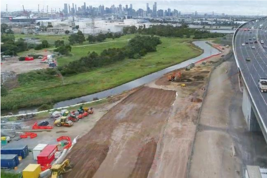
Site preparation to support construction of inbound Hyde Street off ramp and SUP
