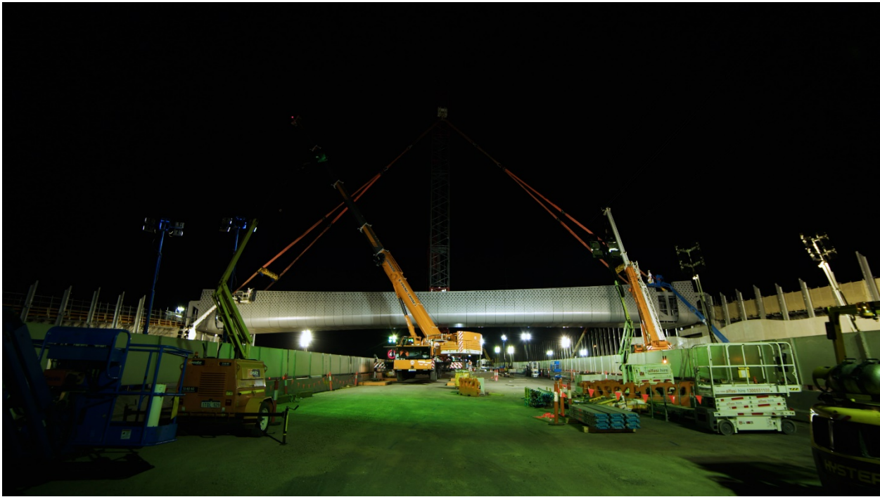
The Muir Street walking and cycling overpass is safely positioned across the West Gate Freeway
