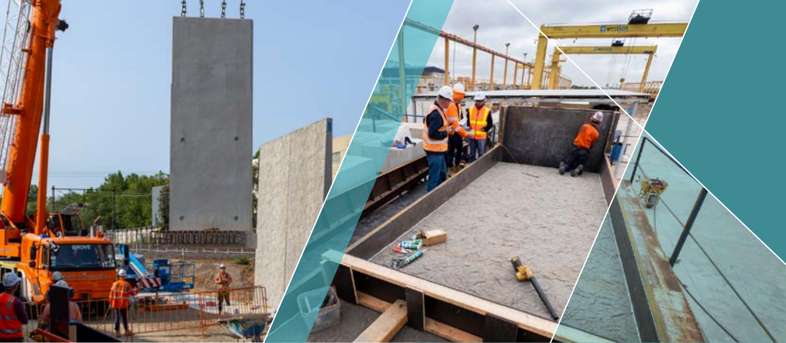
Above left: Retaining wall installation in Tooronga Park. Above right: Casting a section of the retaining wall.
