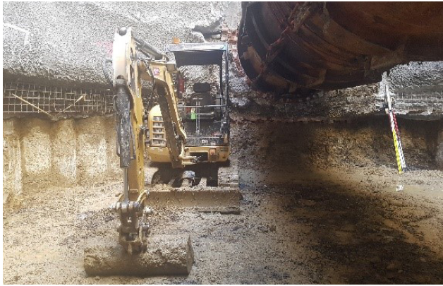
Above: Temporary mechanical flumes (pictured) were installed in the 130-year-old North Yarra Main Sewer to maintain the sewer flow while we completed the diversion. This shows the excavation below the flume.
