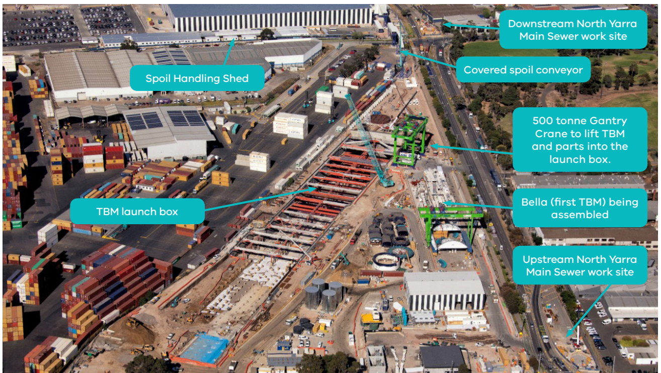
An aerial view of our bustling site on Whitehall Street where the TBMs, Bella and Vida will be launched.
