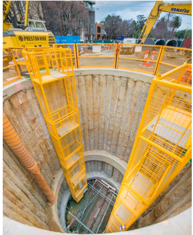
The South Yarra Main Sewer being relocated for the Metro Tunnel Project.
