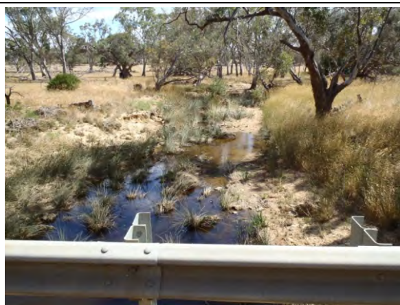
Figure 9: Exposed banks and some bank slumping observed looking downstream from the existing bridge.
