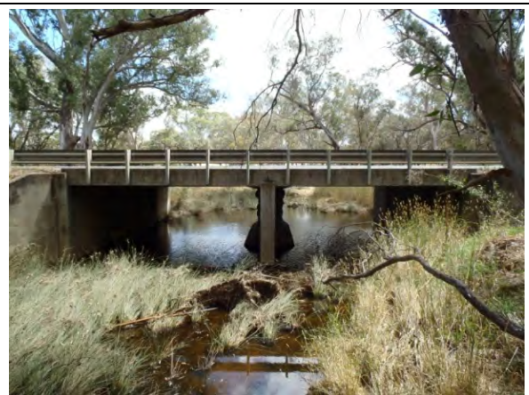
Figure 10: Instream bar observed upstream of the existing highway crossing.
