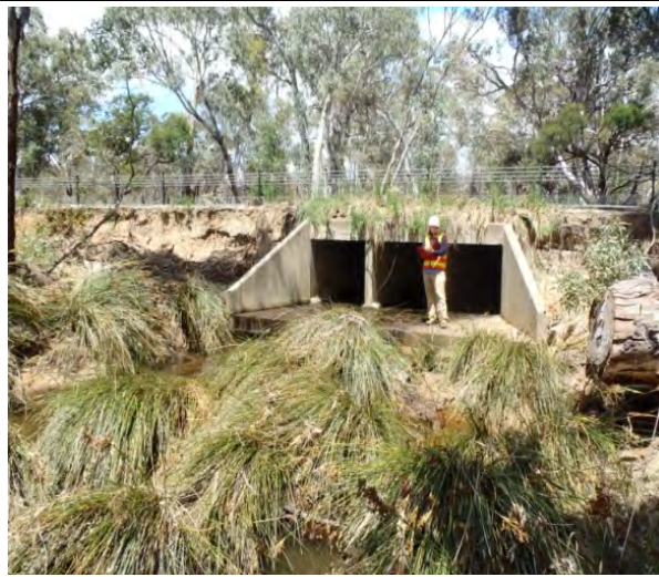
Figure 19: Robinsons Creek, looking upstream, north of the road culverts. N.B. scour behind culvert wing walls and the significant different between culvert and channel invert levels.
