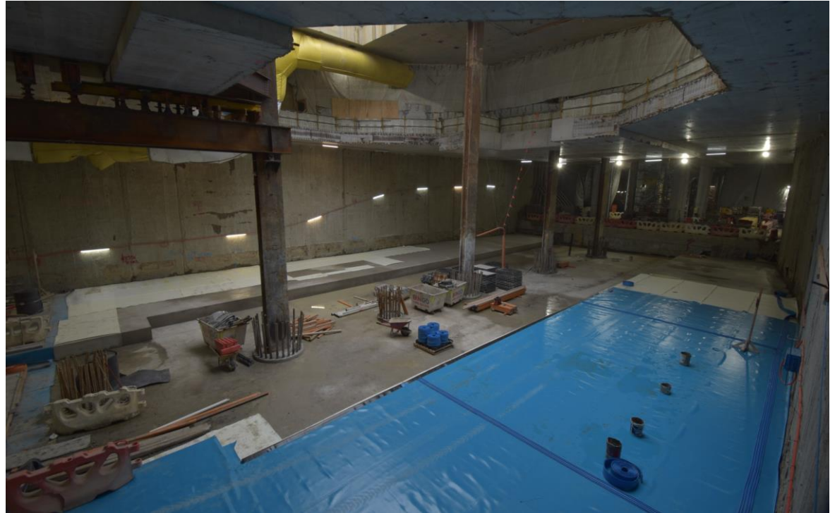
Northern end of the south box – Excavation complete and blinding layer down
