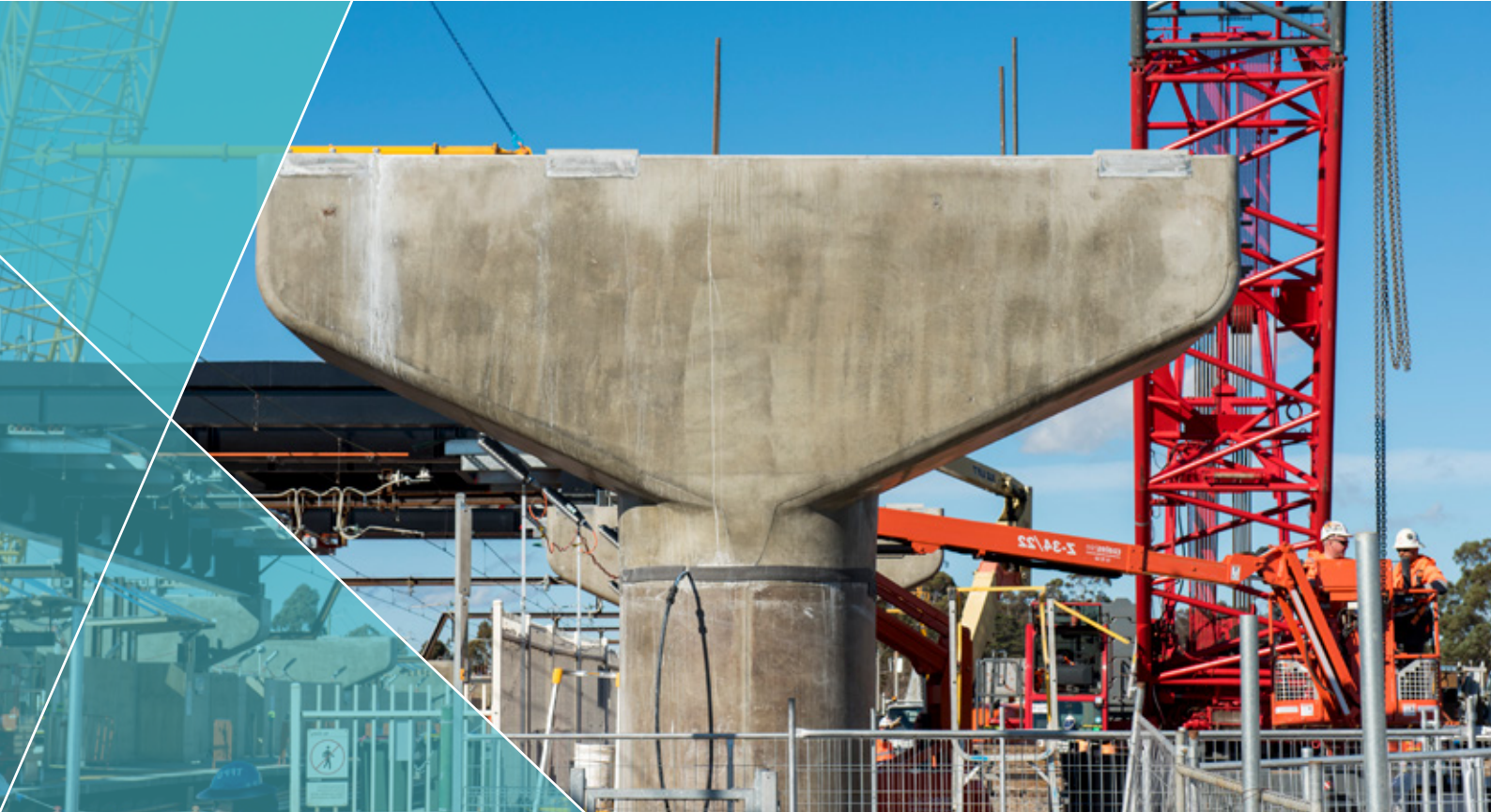
Pier and headstock installation during construction at the Reservoir Level Crossing Removal Project
