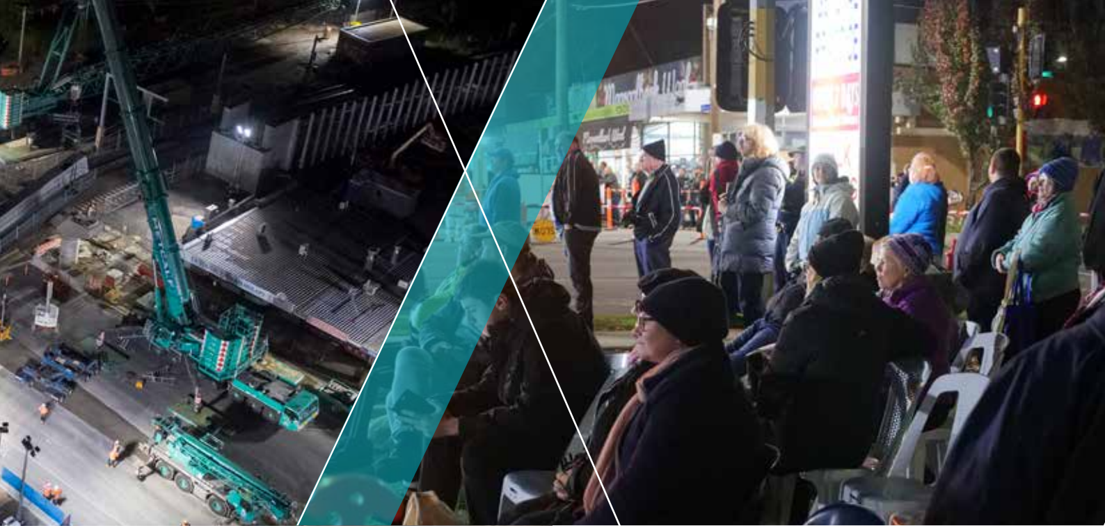
Image 1: Drone footage of the Manchester Road L beams installation; Image 2: A crowd watches on as the beams are lifted into place
