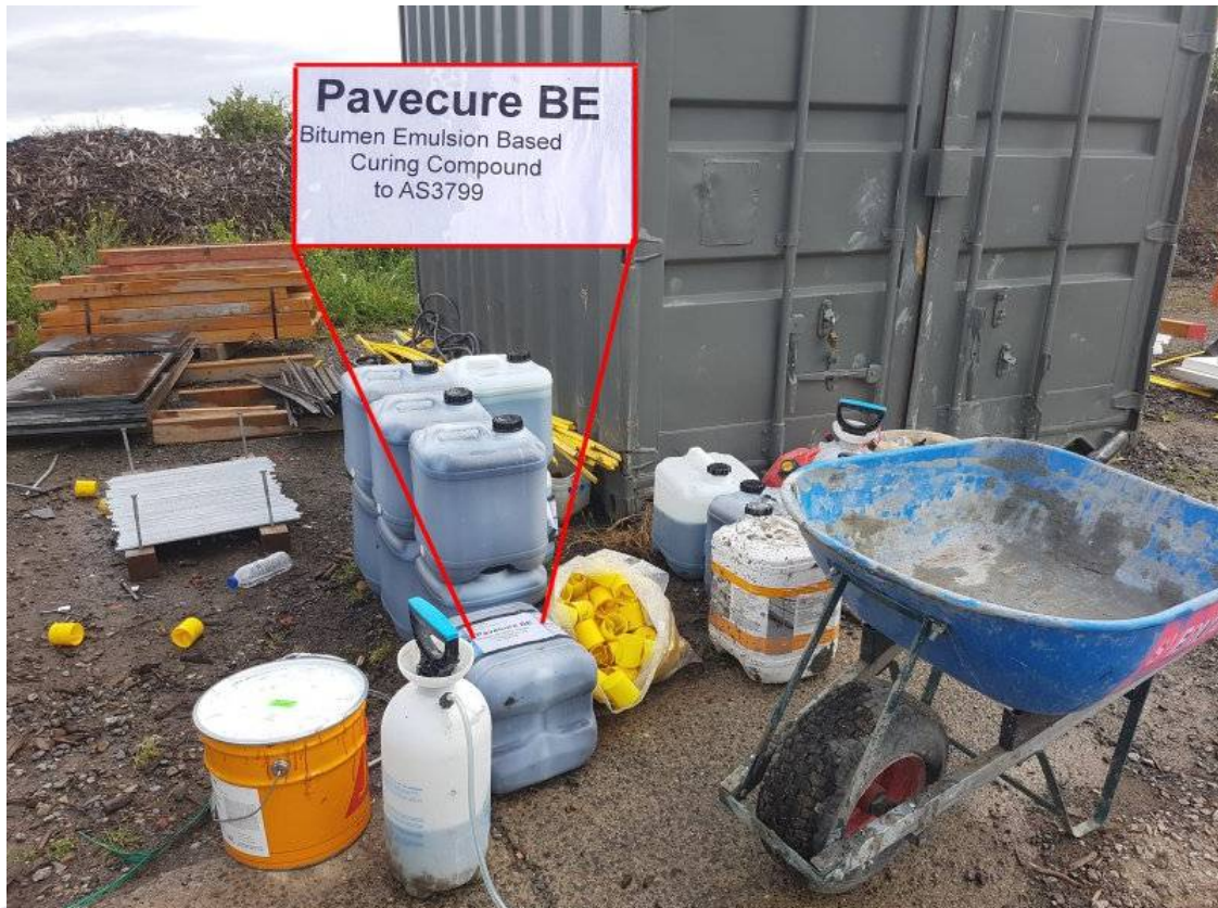
Above: 20L containers of fluids stored on bare soil at the landfill bridging structure works area. A contractor was asked to place these materials in the storage container. This occurred before the inspection of the area was completed.
