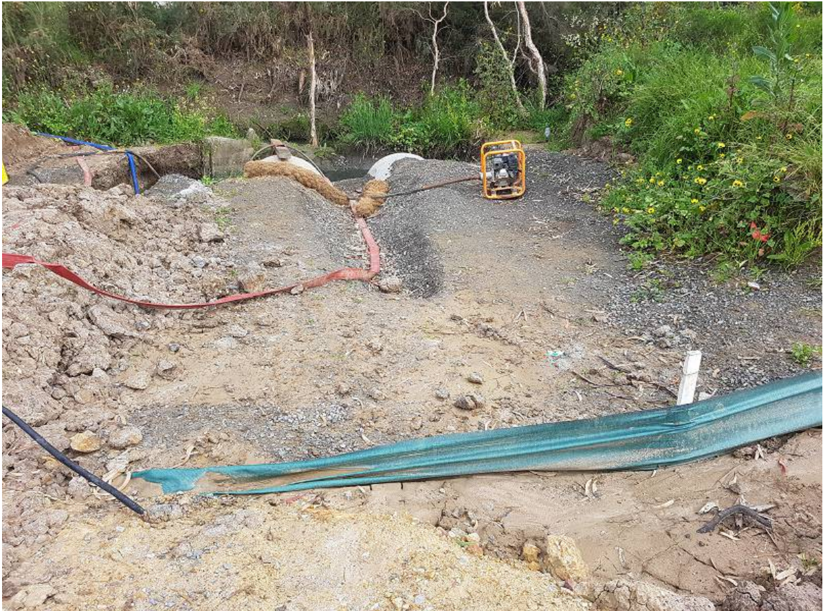
Above: Discharge point into drain approximately 100m south of Centre Dandenong Road.
