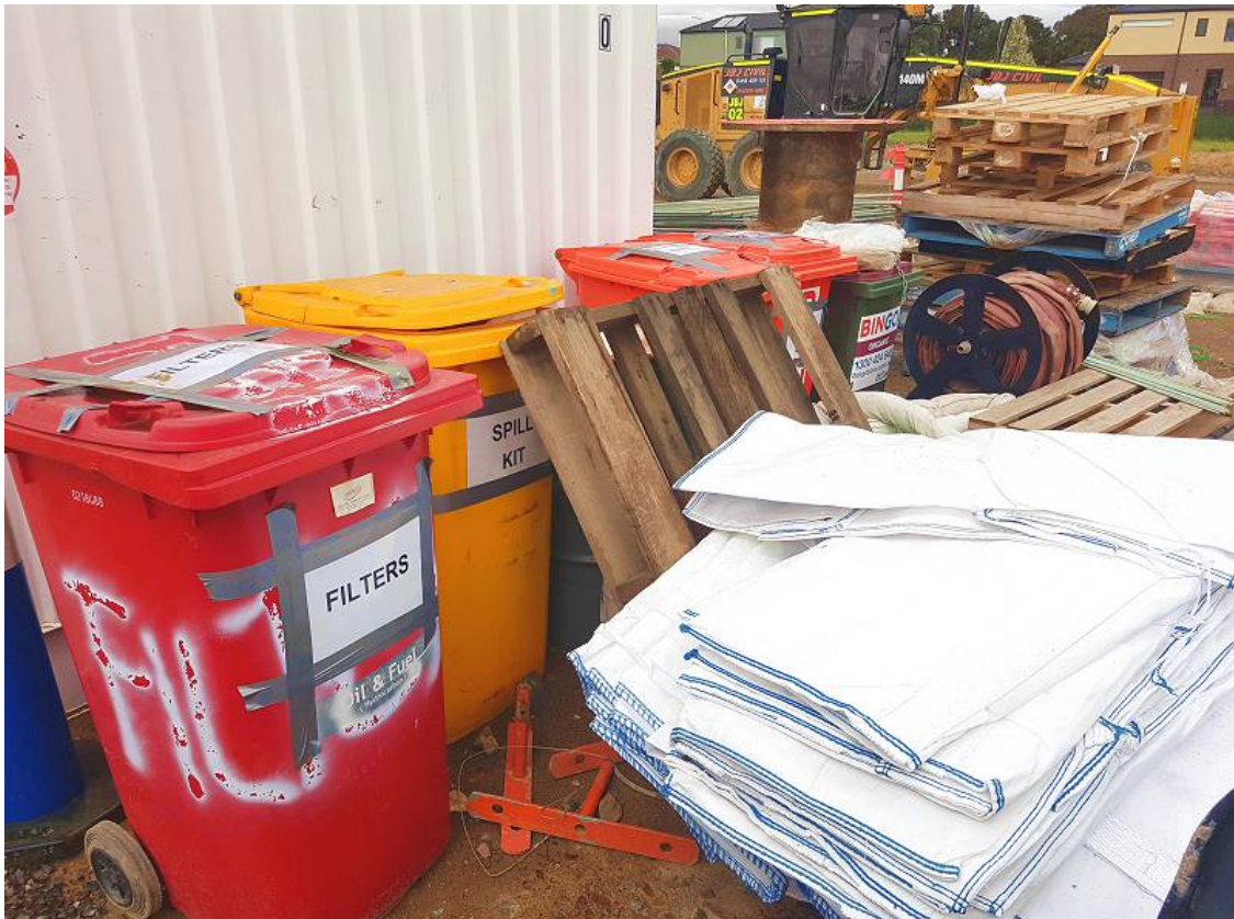
Above: The spill kit and waste bins at the contractor's storage area south of the Waterways piling area were inaccessible due to storage of material against the bins.
