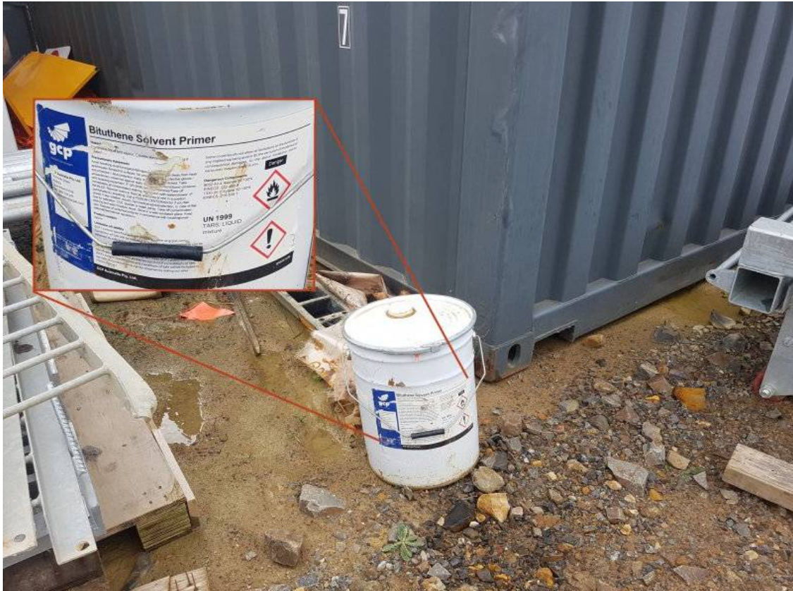
Above: Drum of bitumen solvent primer stored on bare soil at the contractor's storage area south of the Waterways piling area
