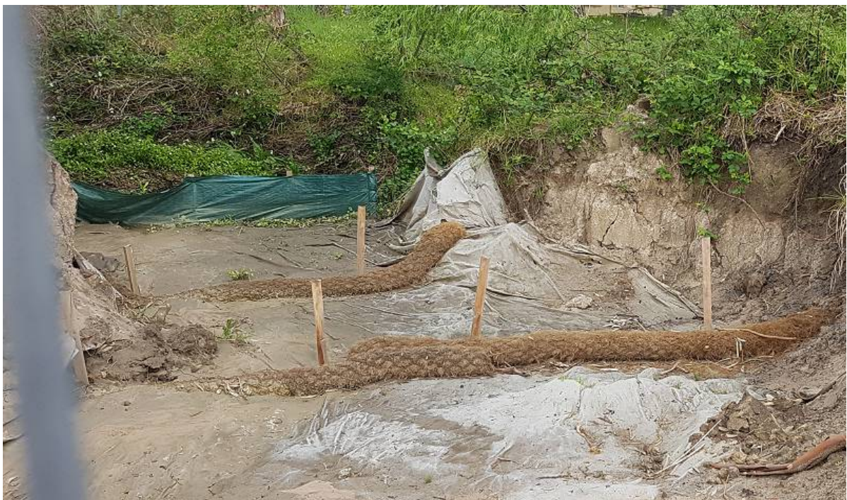
Above: Discharge point into drain approximately 20m south of Centre Dandenong Road.
