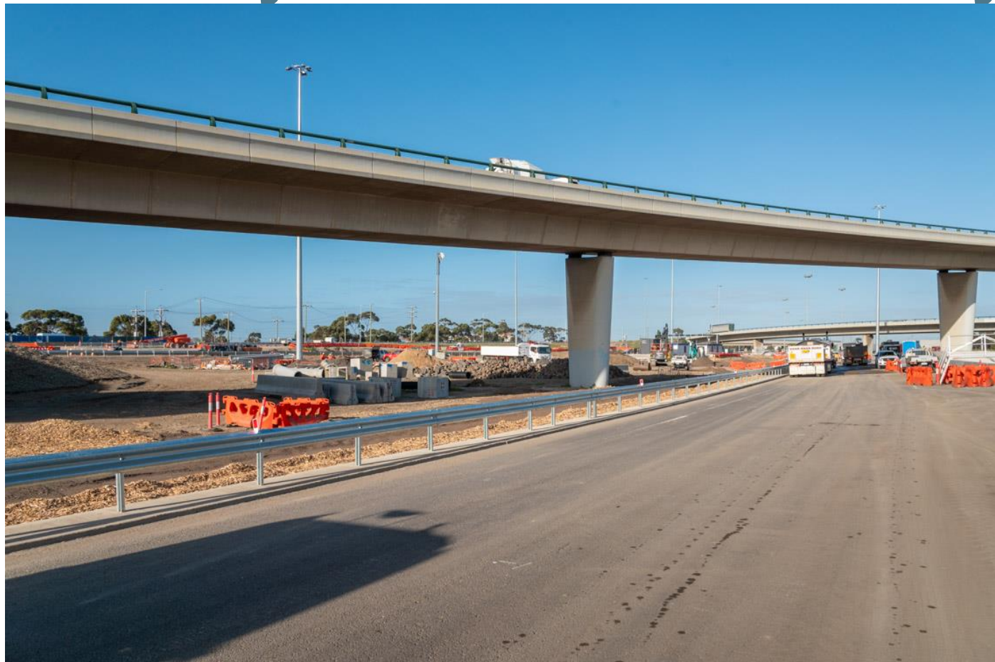
Upgraded pavement for the WGF Outbound to Princes Freeway, this will be used by the Express Lanes from the West Gate Bridge
