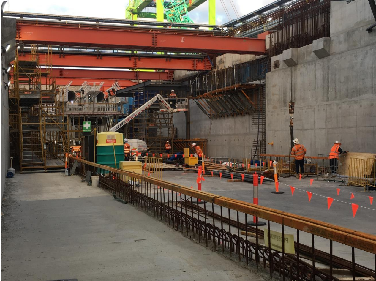
Constructing walls, decks and other concrete elements within the North Portal launch box
