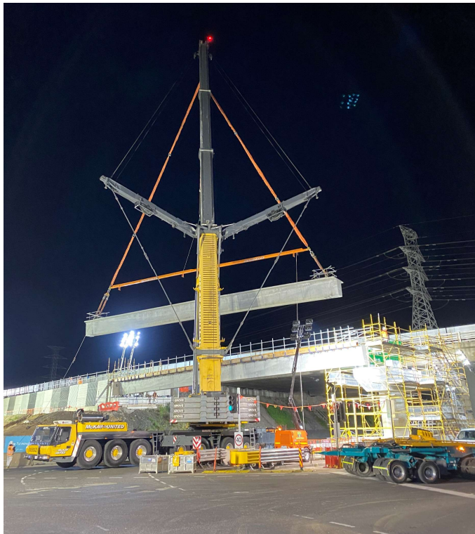
One of six concrete beams being lifted into place on Williamstown Road
