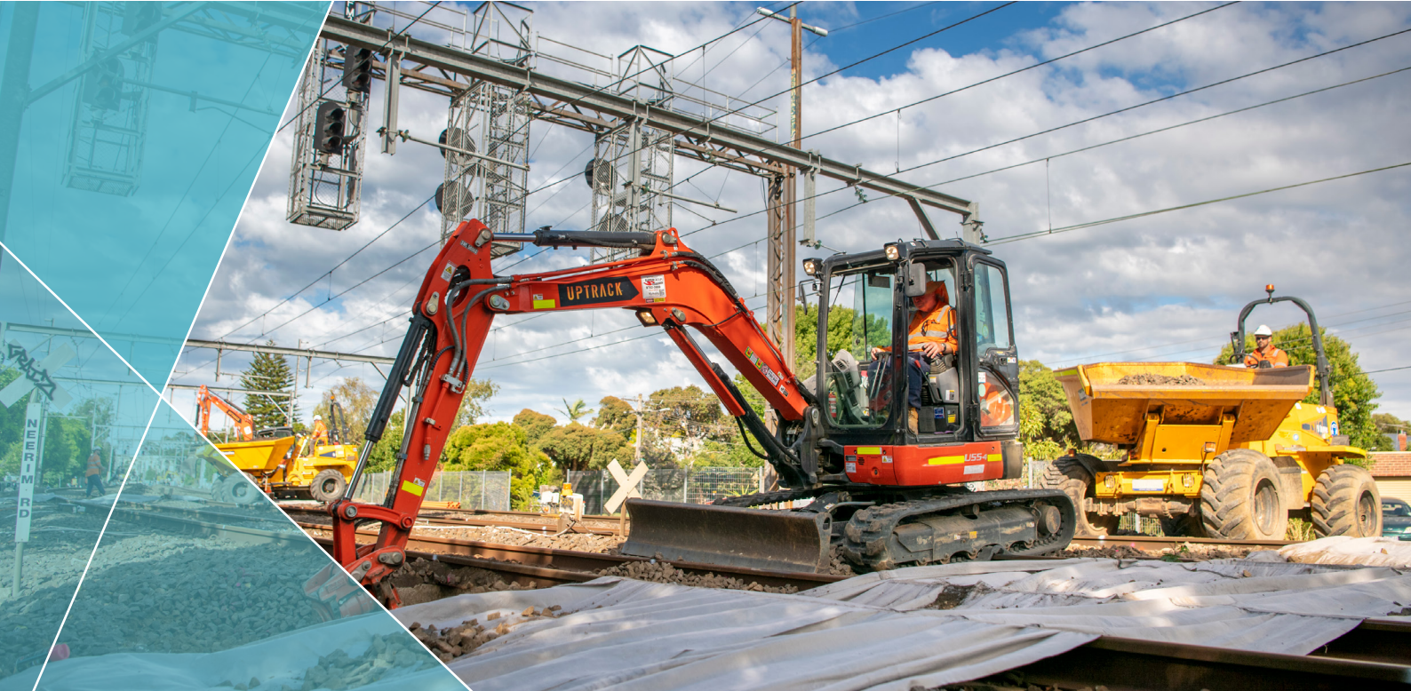
Foundation works have been well underway to prepare for digging the one-kilometre trench
