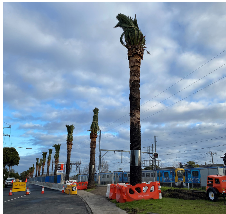
Canary Date Palms sporting an up-do while we prepare them for removal and safe-keeping until they can be replanted
