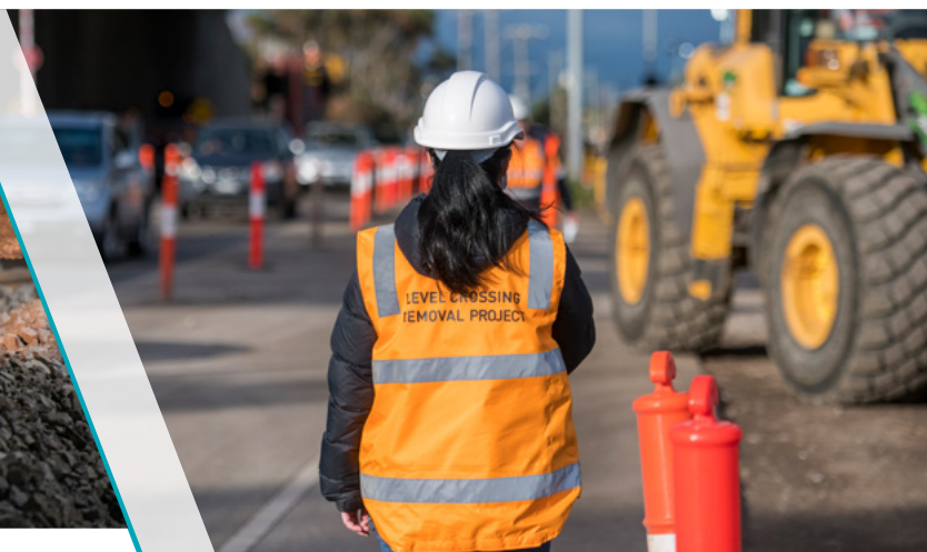
A worker navigates the works adjacent to Forrest Street during our winter construction blitz
