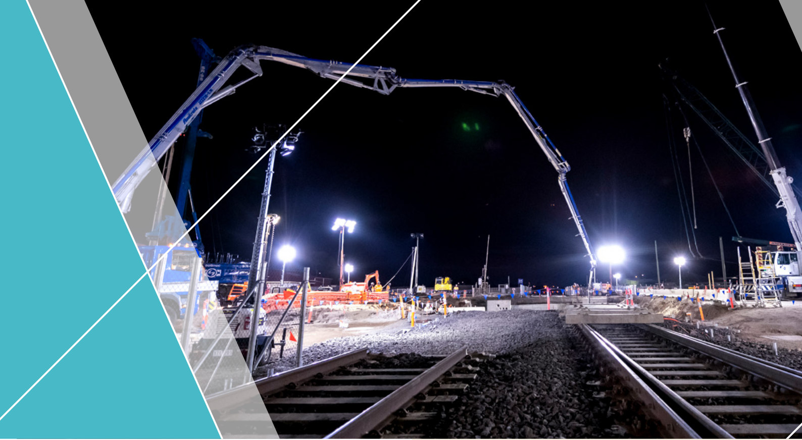
A concrete pour is completed in the rail corridor on Robinsons Road
