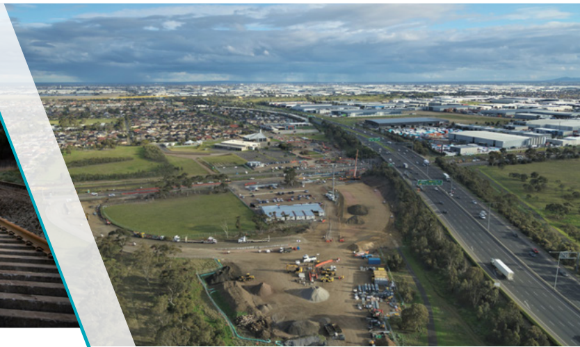
A sneak peek at the new road alignment under construction north of Forrest Street
