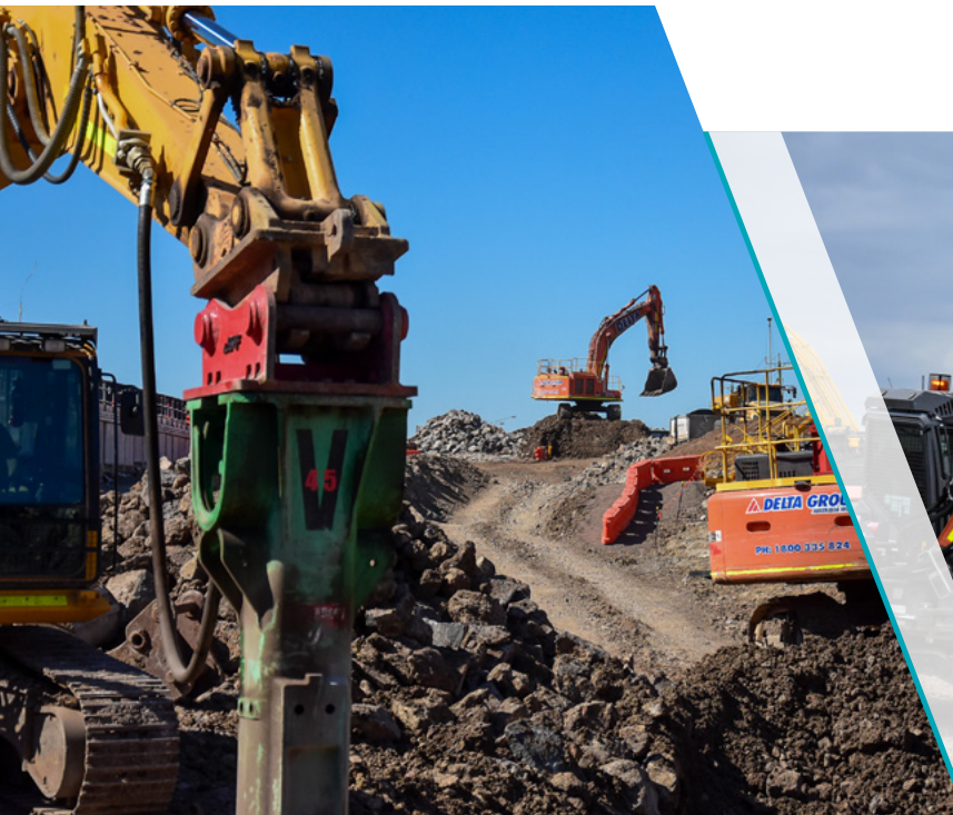
To build the new road at Robinsons, we need to remove over 42,000 cubic metres of dirt and rock
