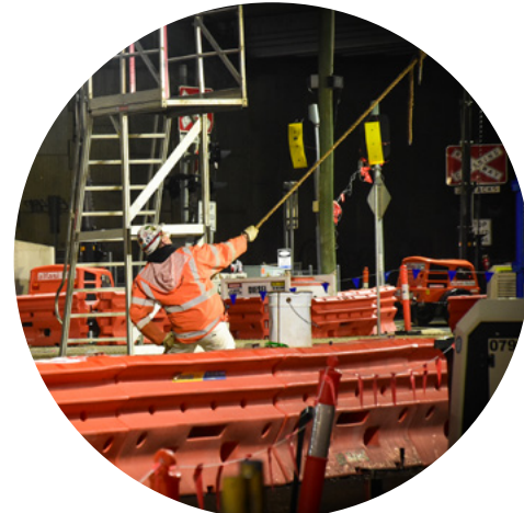
Top: The view of Forrest Street from the new road bridge looking towards the city Bottom: A worker guides the beam into place using secured ropes
