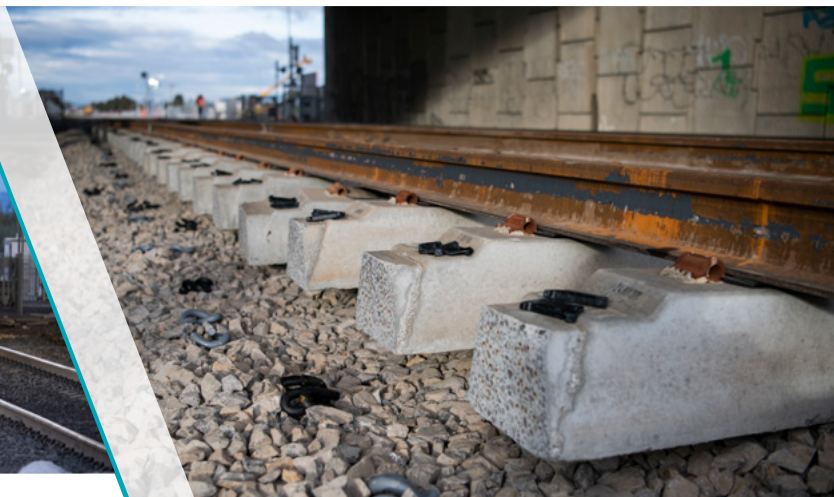
Up close and personal to the newly installed rail line on Fitzgerald Road
