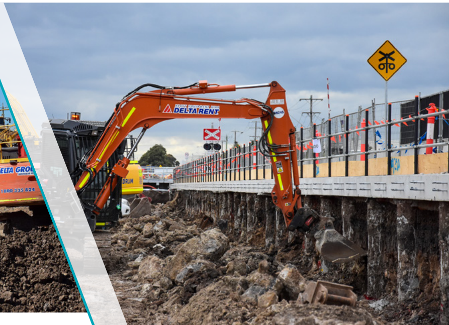
The amount of dirt and rock removed is the equivalent of nearly 17 Olympic size swimming pools
