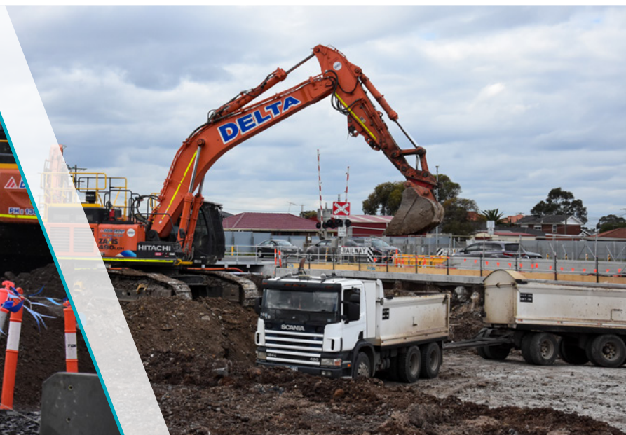
Excavation of the road is taking place next to the new rail bridge adjacent to Robinsons Road
