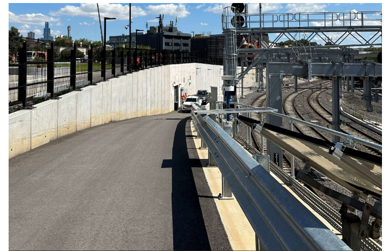
South Yarra traction power substation
