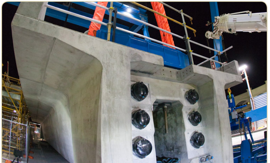
The finished span once the steel cables have been stressed, the end caps installed and grouting completed.
