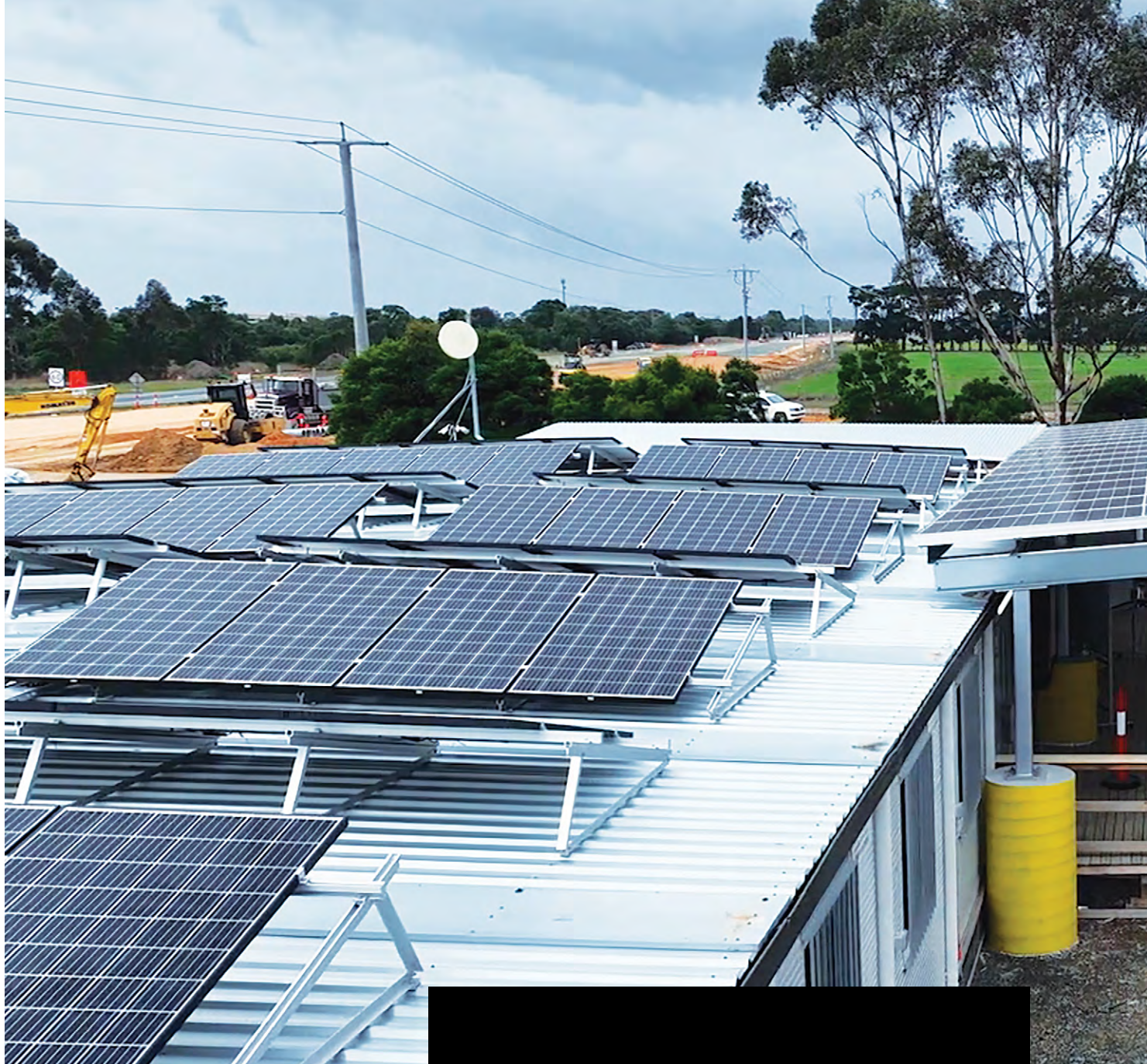
Image: Site solar array at the Princes Highway East – Kilmany upgrade project.
