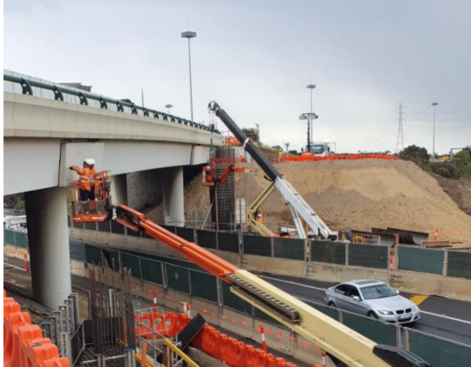
Widening works on Bridge 10 (Western Ring Road through to West Gate Freeway)
