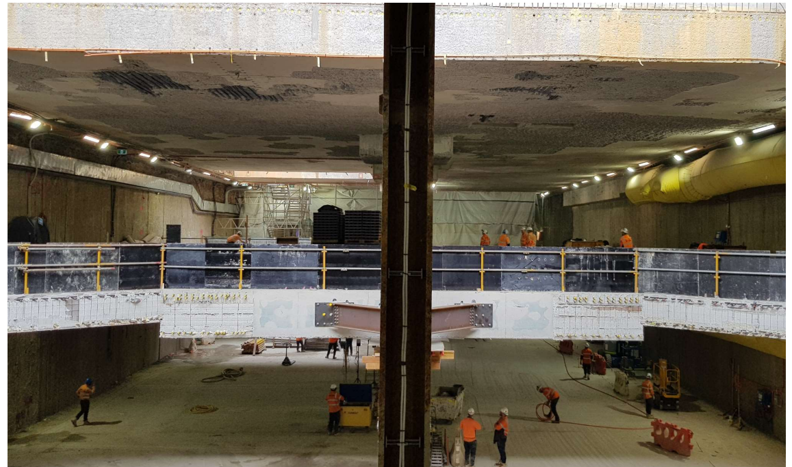
Above and below the newly poured concourse level, prior to stage 2 breakout
