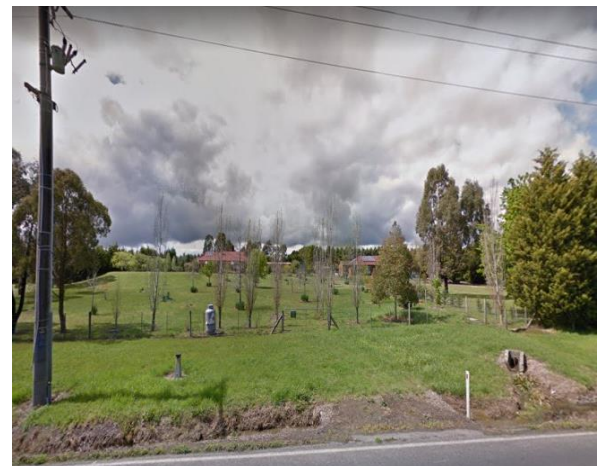
Plate 64: Culvert and services in eastern road reserve of Yan Yean Road, Yarrambat (Minos 18.12.2017)
