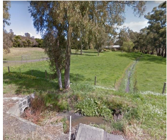
Plate 62: Channelization of minor waterway crossing Yan Yean Road, north of Youngs Road, showing culvert and underground services (Minos 18.12.2017)
