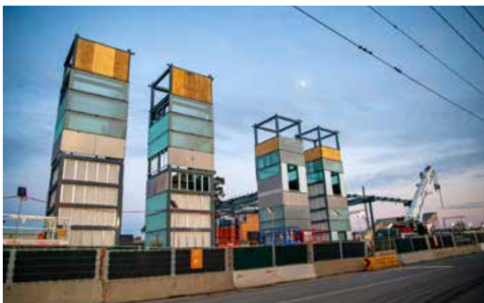
The four station lift shafts were delivered and fitted out on-site before being craned into place. Each lift shaft is 13.3 metres tall.
