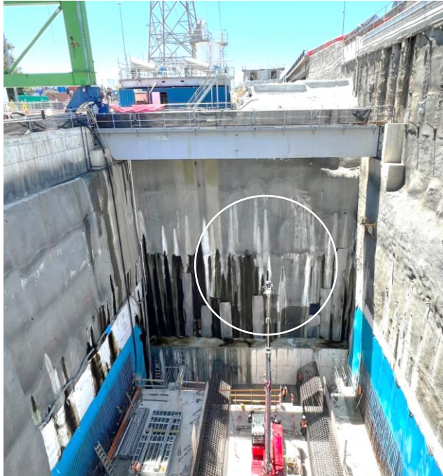
Headwall at Southern Inbound Portal and concrete cradle in the 30m deep retrieval pit.
