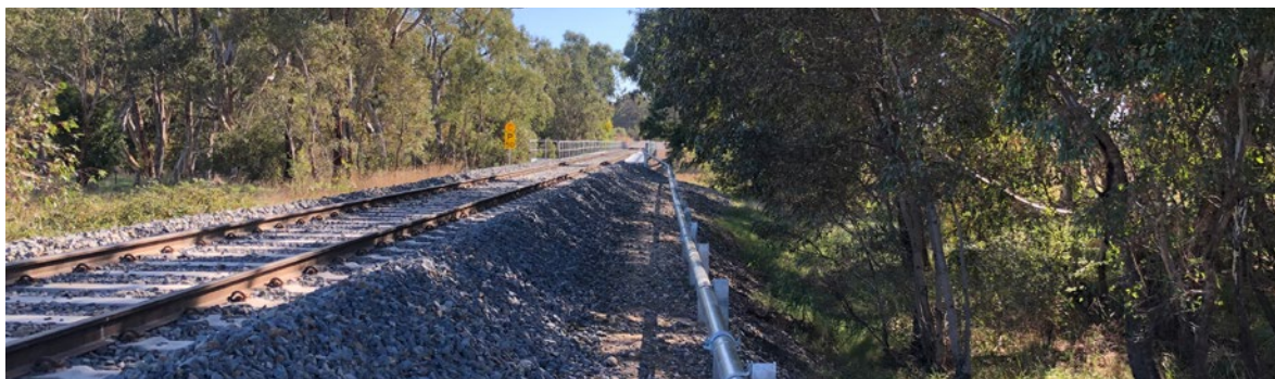
Figure 4: GPOP (Galvanised Pipe on Post), installed in the Shepparton Rail Corridor as an above ground signalling solution to mitigate the vegetation removal required for trenching or boring
