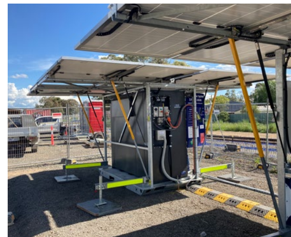
Figure 10.1: Makinex Hybrid Power system at Nagambie Compound
