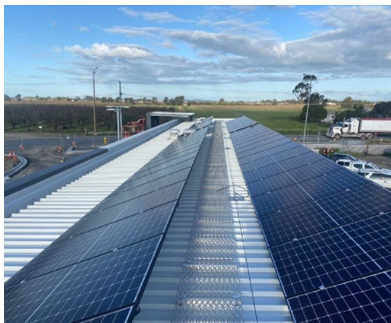
Figure 9: Solar Panels at Shepparton Stabling Yard
