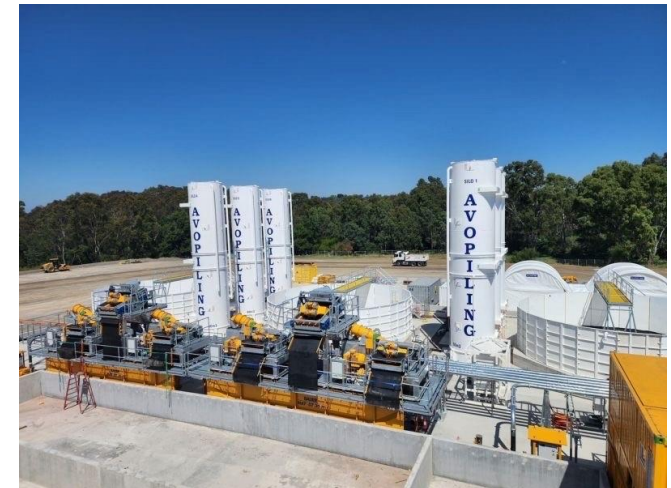
Image: An example of a bentonite plant to be installed to enable TAS construction.
