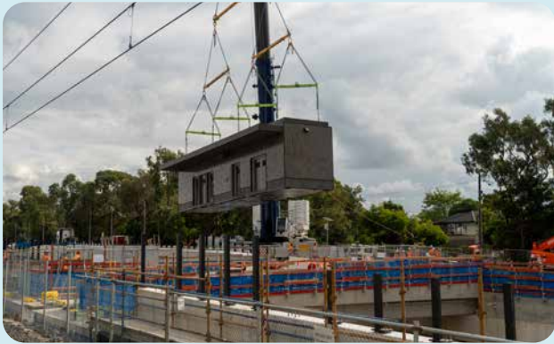
Four Ringwood East Station buildings were built off-site and delivered and craned into position.
