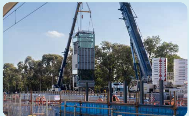
Four lift shafts for the two station entrances were delivered and lifted onto site earlier this year.
