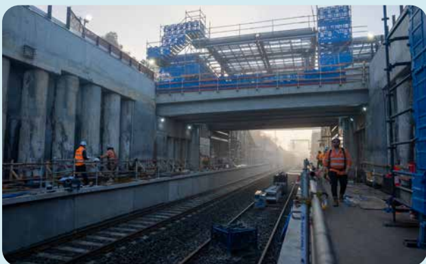
Almost 2km of new rail track has been laid as part of the new rail trench.
