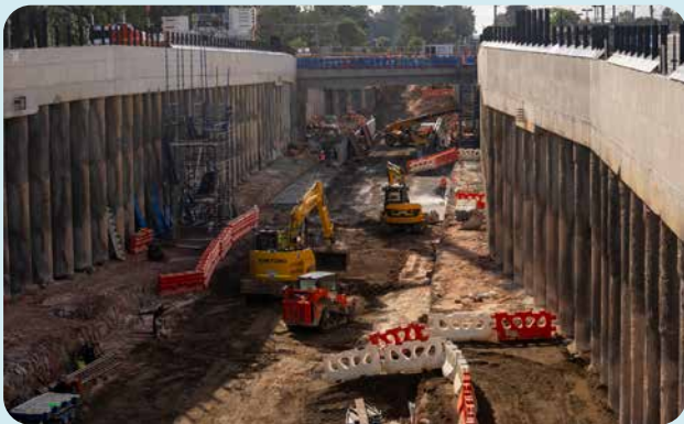
Approximately 65,000 cubic metres of dirt was excavated to build the 650-metre-long rail trench.
