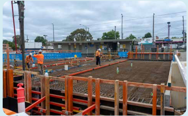
Where possible, works to build the new station and rail trench were done 'offline' next to the existing station and train line while trains were still running.
