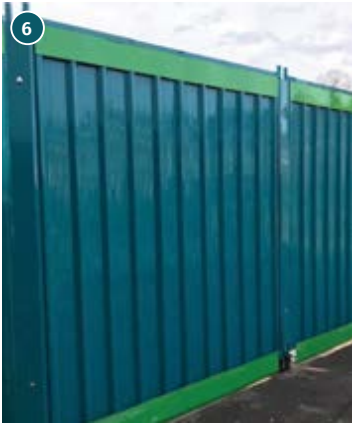
USE TEMPORARY FENCING AND HOARDINGS THAT ARE VISUALLY RECESSIVE (SOURCE: SAFE FENCE)
