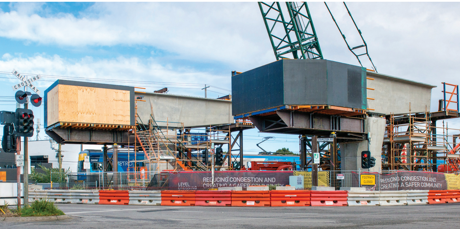
Installation of large extensions on piers (called haunches) at Clayton Road level crossing.
