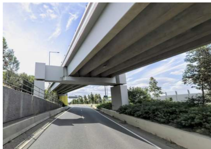
Figure 37: Example of portal piers at Tullamarine Freeway – Mickleham Road interchange inbound entry ramp
