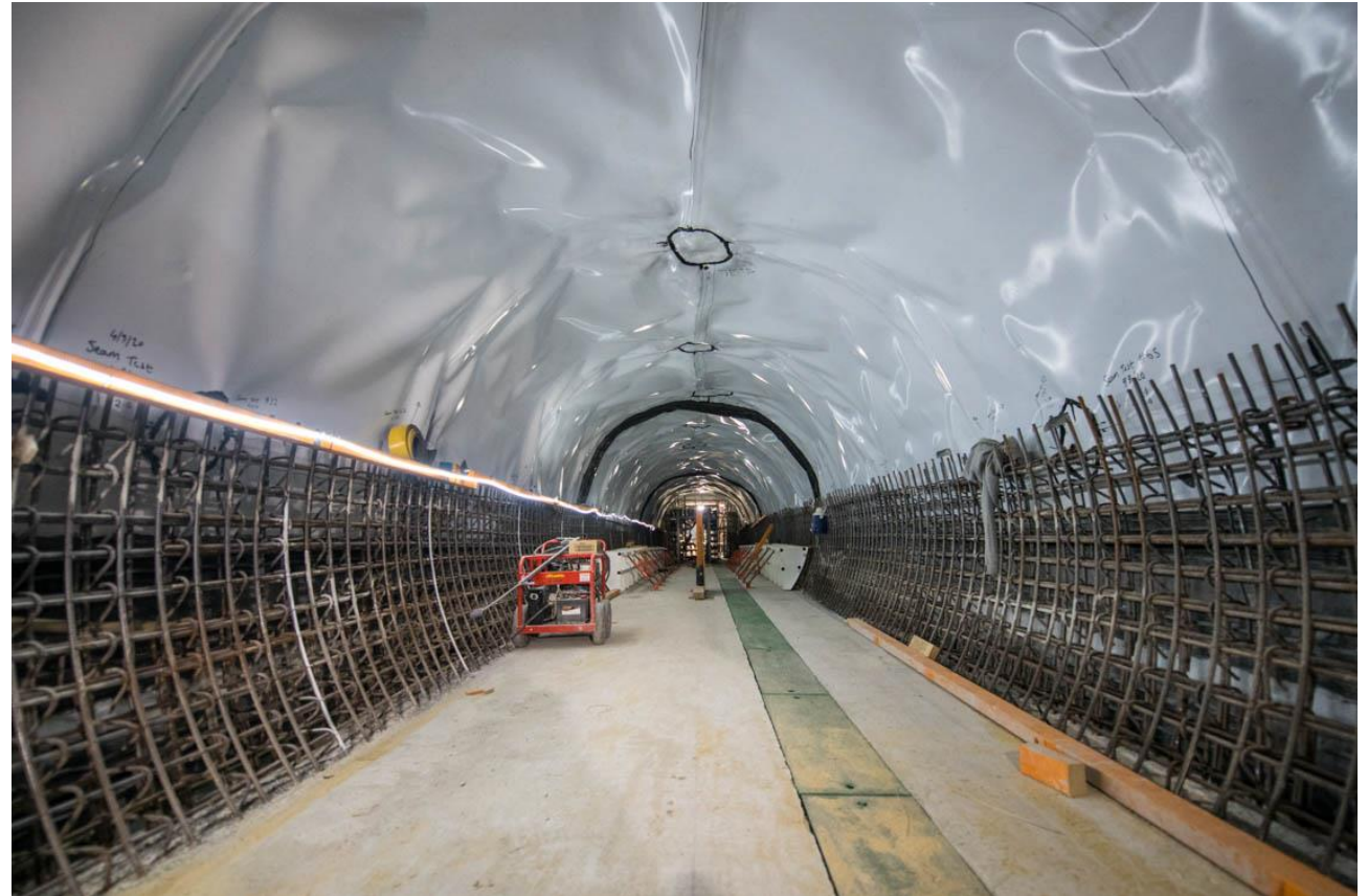
Partially constructed cross passage in Western Precinct, waterproofing membrane and steel fixing
