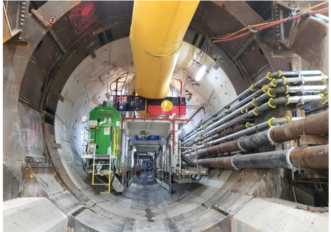
TBM Alice leaves the Anzac Station on her way to Town Hall Station
