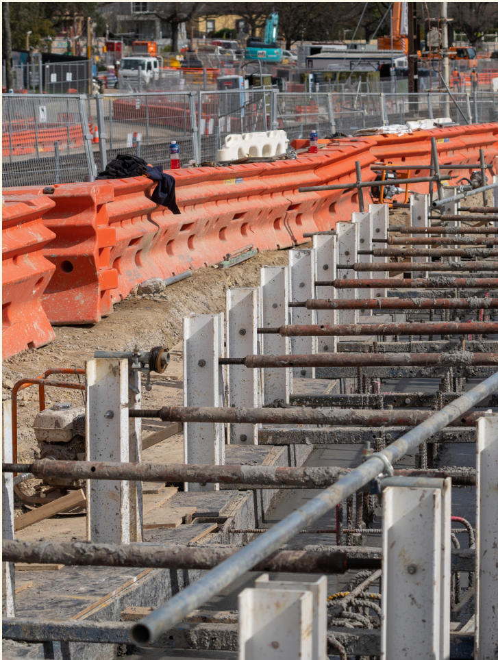
Installing the capping beam that forms the top of the trench wall.
