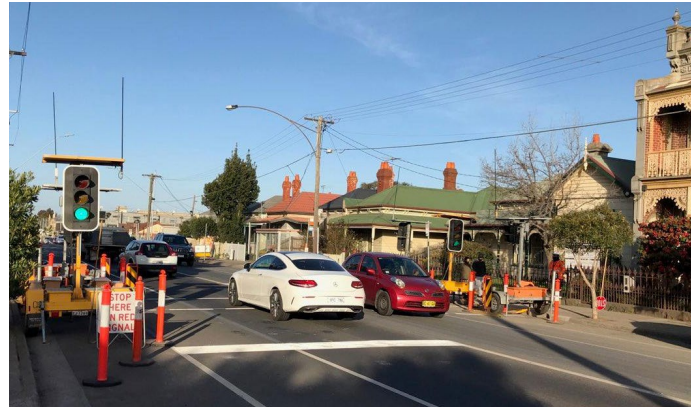
Solar Powered Traffic Lights
