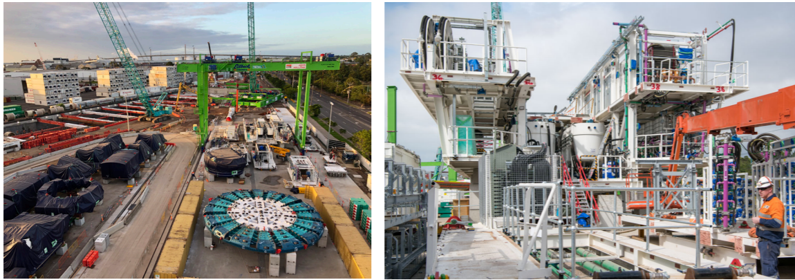
L-R: Birds eye view northern portal site and the first TBM gantry (tunnel building factory) awaiting assembly.
