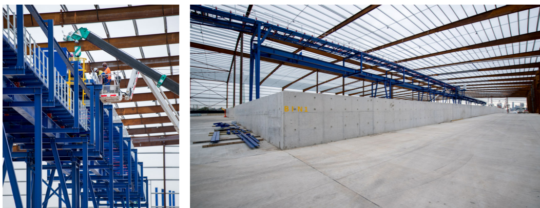
Spoil handling shed and conveyor taking shape on the site at 221 Whitehall Street.
