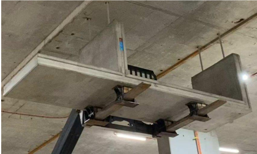
Over track exhaust system segment
