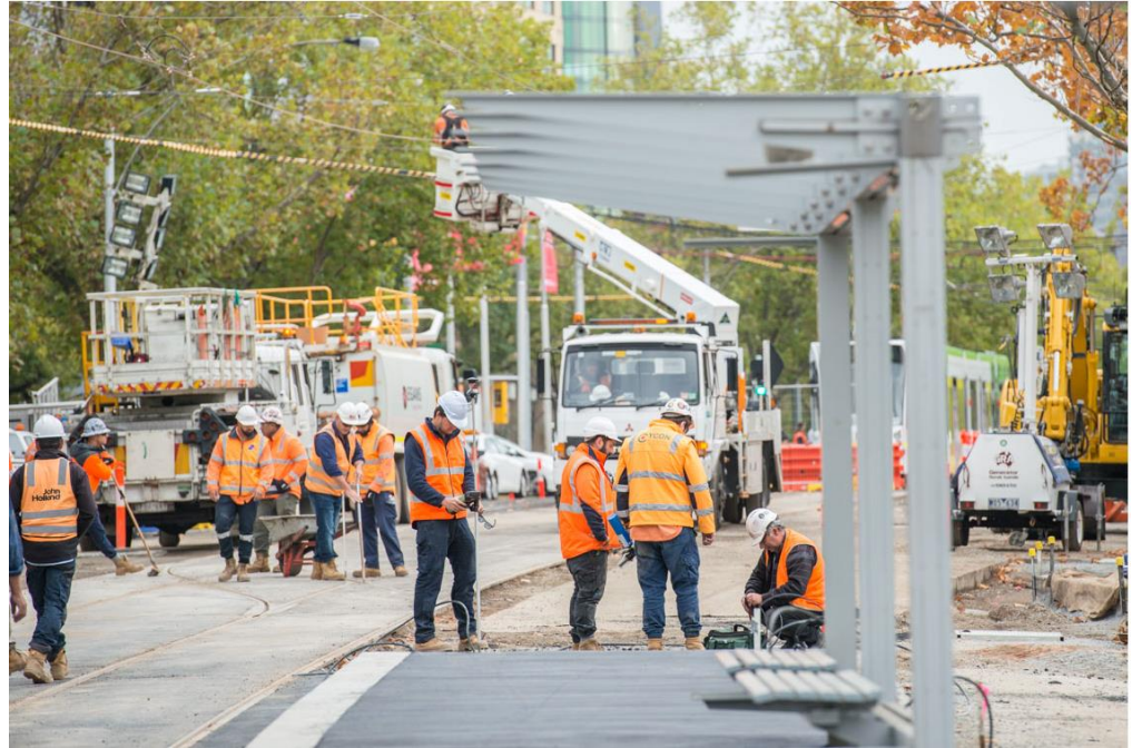
Current Park Street Tram Stop on St Kilda Road installed in 2018 to be removed during 2022 occupation
