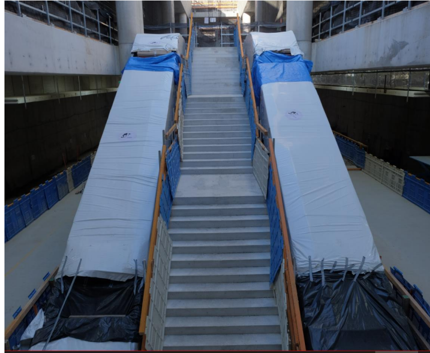
Recently installed stairs and escalators at Arden Station
