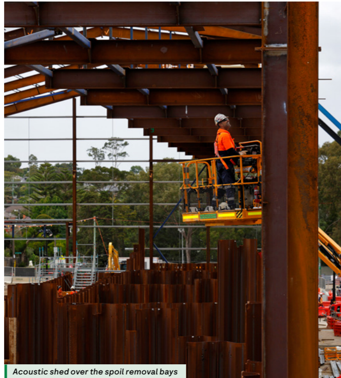
Acoustic shed over the spoil removal bays
