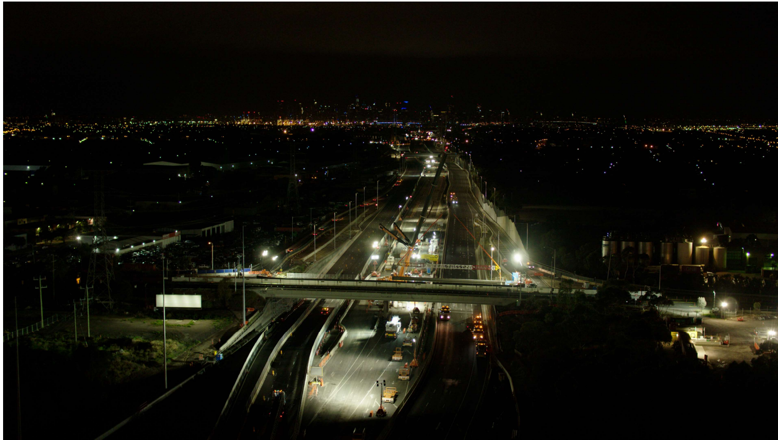
Lifting the new concrete beams into place which will become the new bridge – end of January 2021
