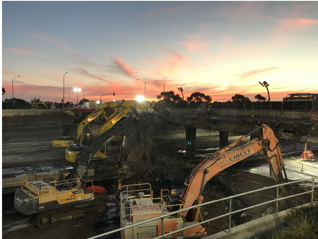
Demolition of the eastern section of the Grieve Parade bridge between 6 – 11 January 2021
