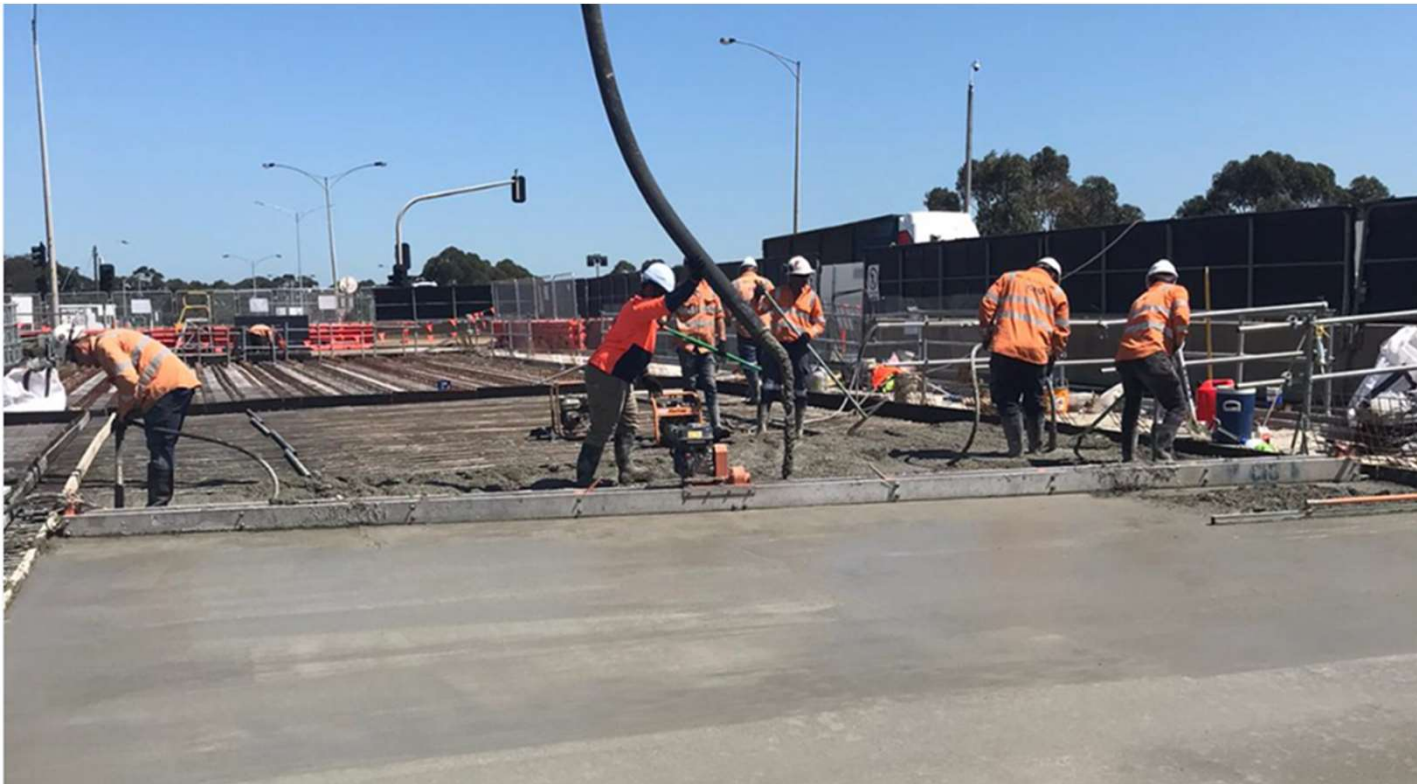
Pouring concrete on the newly installed concrete beams to create the surface of the new bridge – early February 2021
