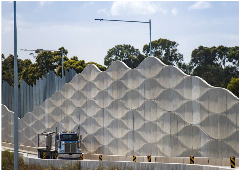
New noise walls installed along the Grieve Parade outbound exit ramp, Brooklyn
