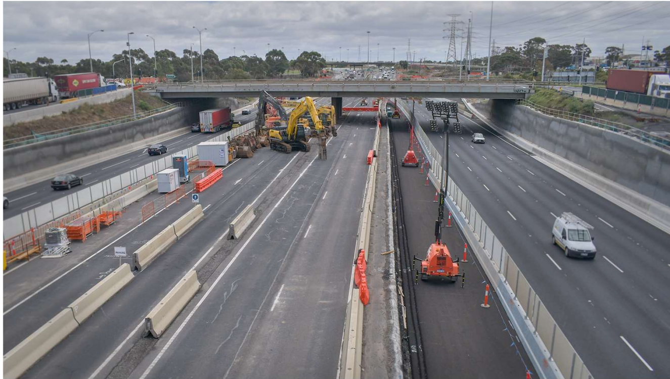
Demolition of the eastern section of the Grieve Parade bridge between 6 – 11 January 2021
