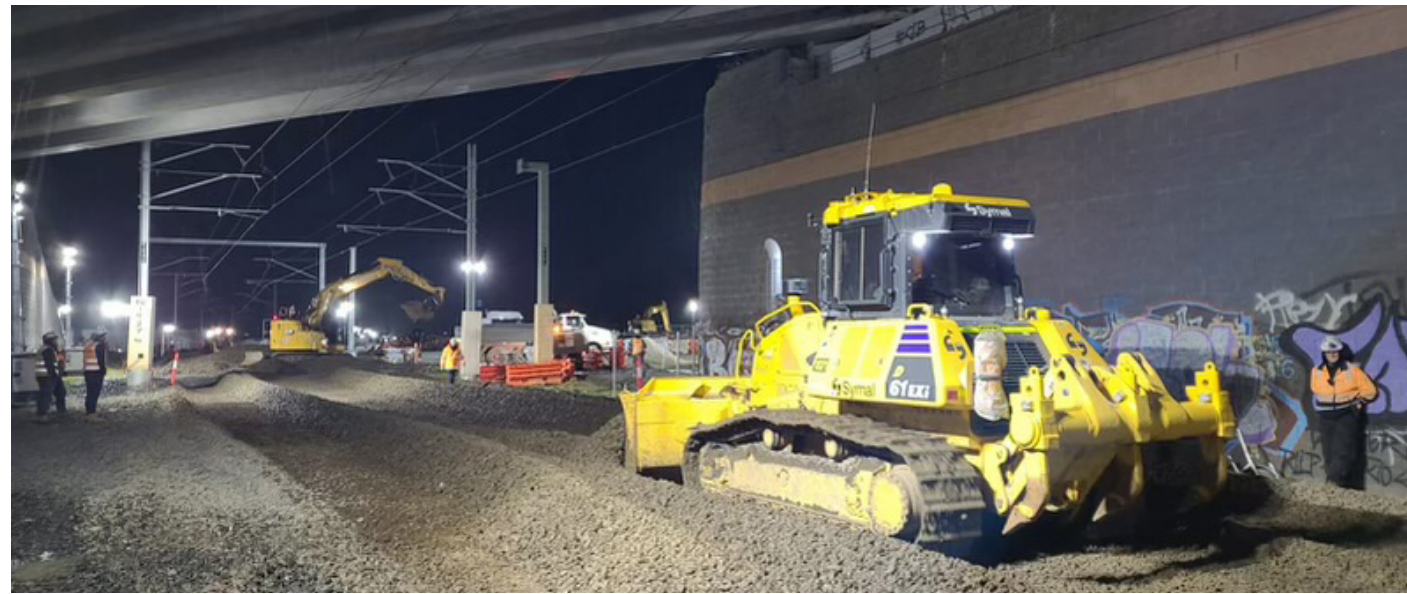
Renewing ballast and soil from underneath the rail line at East Pakenham
