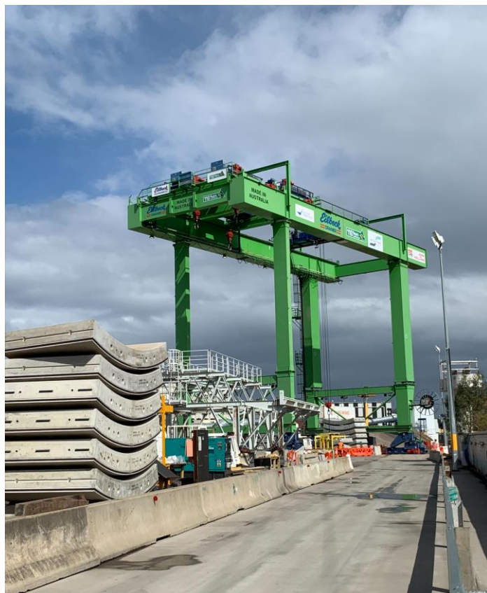
Gantry crane installed that will retrieve tunnel boring machine as it exits the portal. Williamstown Road closures in place in November
